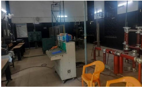
High Voltage Laboratory
